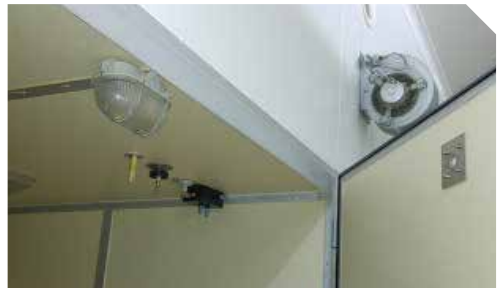
A hole drilled in the door and protected with a metal plate allows the insertion of the calibration probe close to the temperature sensor.
