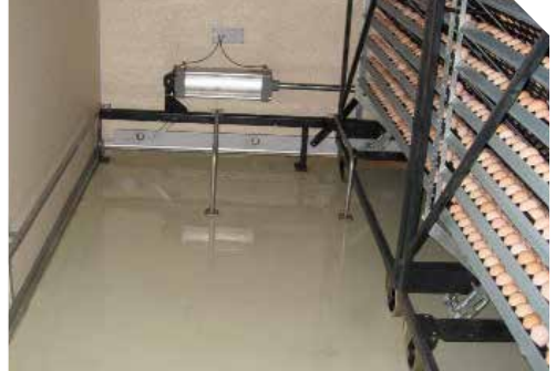
Standing water on the floor of a single stage setter at the end of the sealed period.
