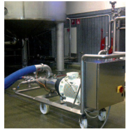
HYGHSPIN as mobile unit for tank unloading.
